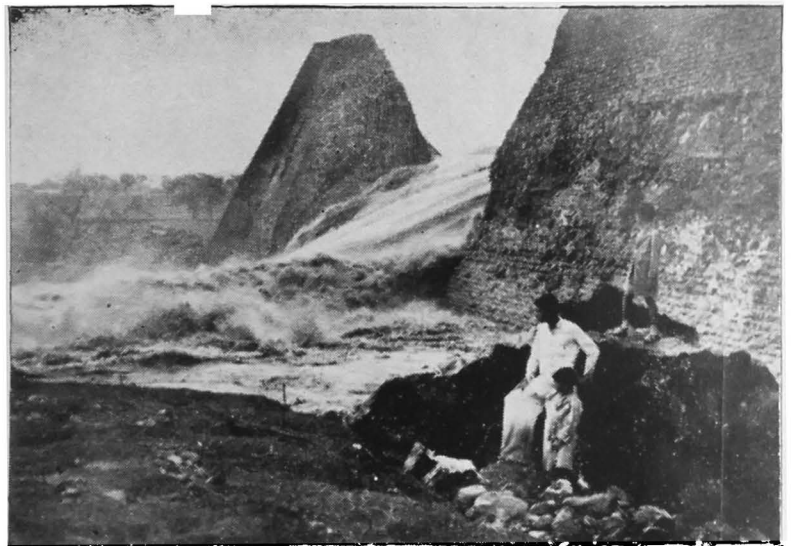
The Breach in the Khadakwasla Dam ( 12th July 1961 )
