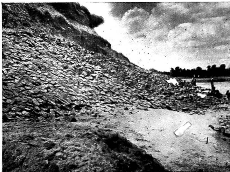
Photo No. 423 : The damaged part of pitching at the North West Corner of the fort wall.
