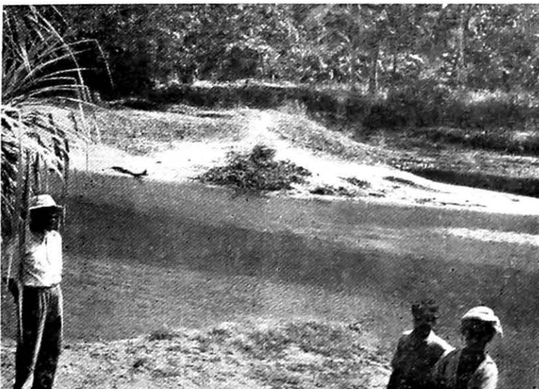
Photo No. 761-The site for an earthen bund at M which is constructed across the cold weather channel to divert water to a small canal
