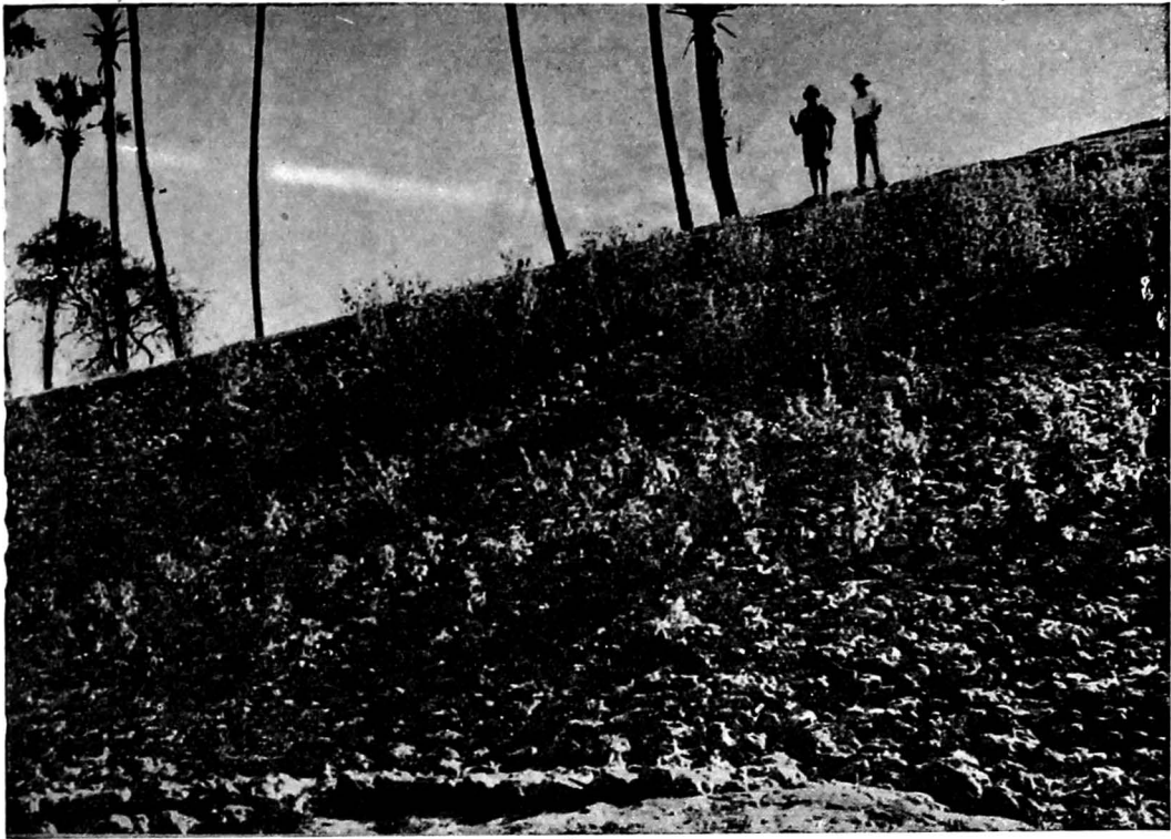
Photo No. 5573—Gautami right bank showing steep clay bank (pitched with stone.) mile 15/2.
