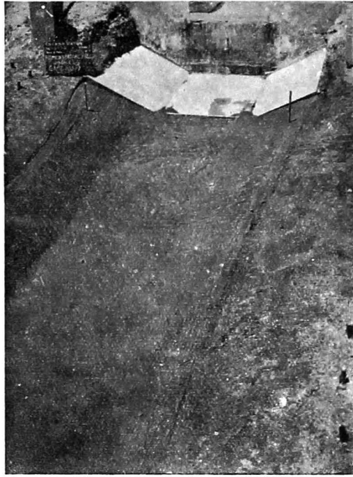
Photo No. 5632 - Looking upstream, shows negligible scour of bed and sides with a standing wave formed at the downstream edge of sill
