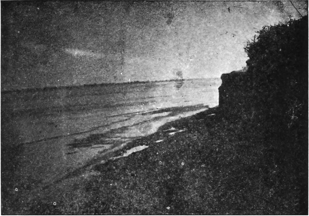
Photo No. 5577—Gautami river 200' Ft. above right abutment showing steep scoured bank looking downstream.
