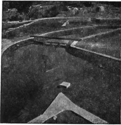
Showing the 300 ft. wide cut from Bennihalla to Radihalla with the Bridge in background.
