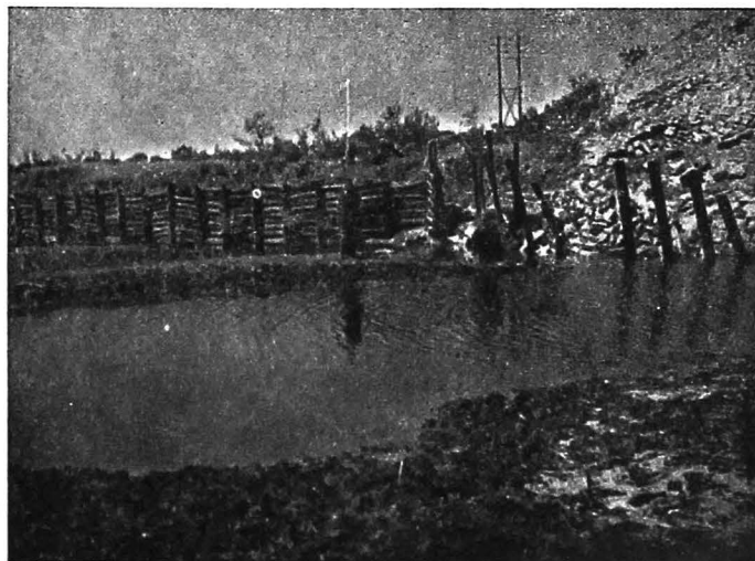
Photo No 5529—A close-up of the standing sheet piling; some piles were pushed out of vertical position by the slipping of apron
