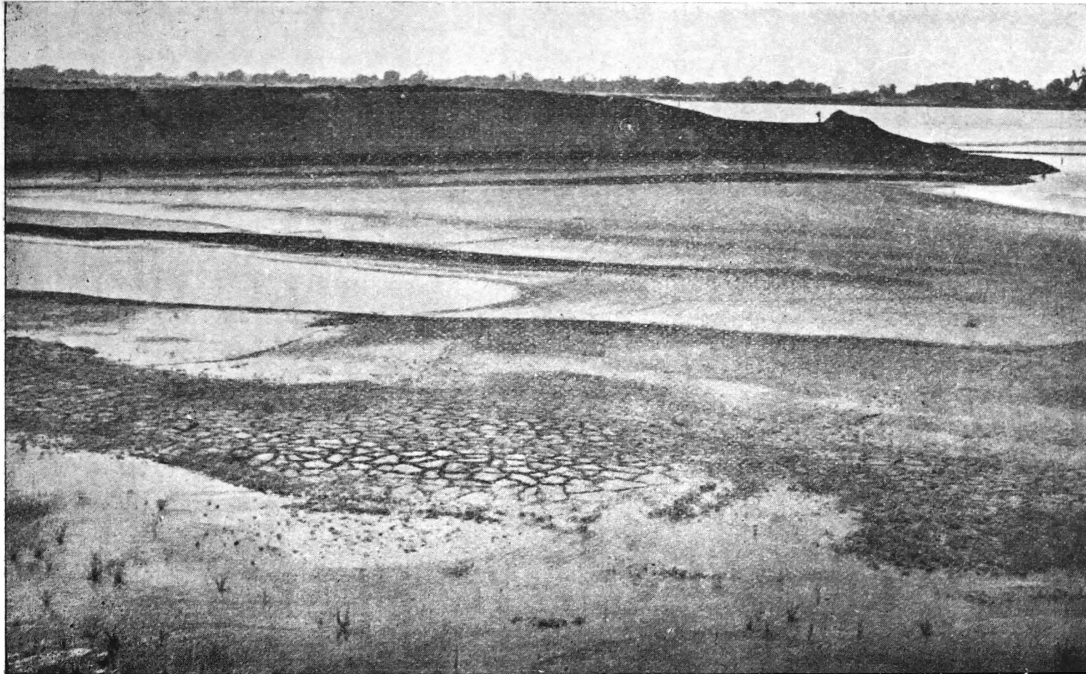
PHOTO No. 5481 Looking downstream from left bank showing the damaged nose of the Khannagar Spur. Note also silting in the foreground, where previously there was a deep water channel.
