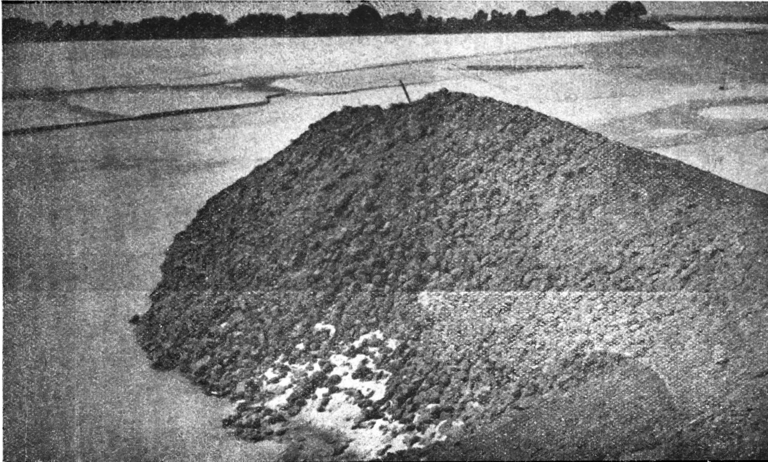
PHOTO No. 5486 Showing a close view of the damaged nose of Khannagar Spur. Taken from the downstream slope of the Spur looking towards the nose.
