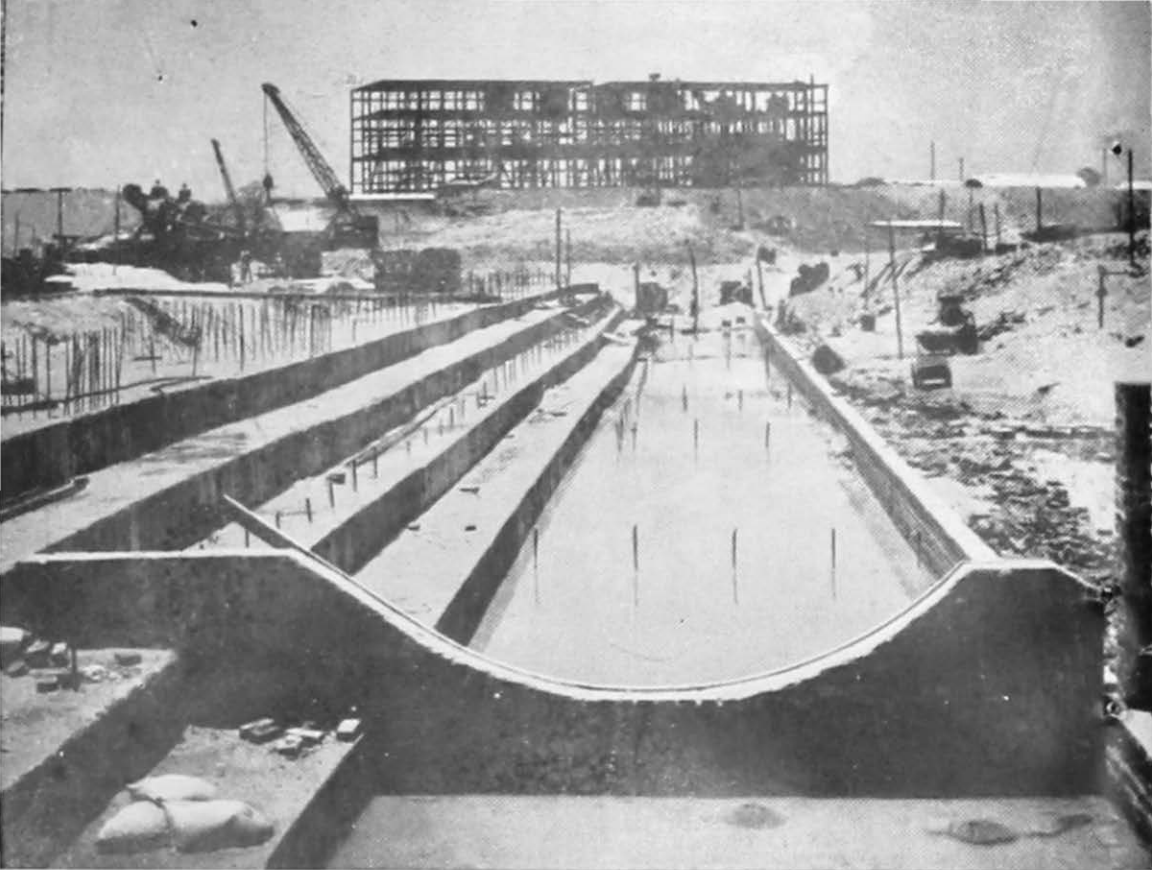
Damodar Valley Project. Construction of the barrage across the river at Bokaro with the steel structure of the power station in the background
