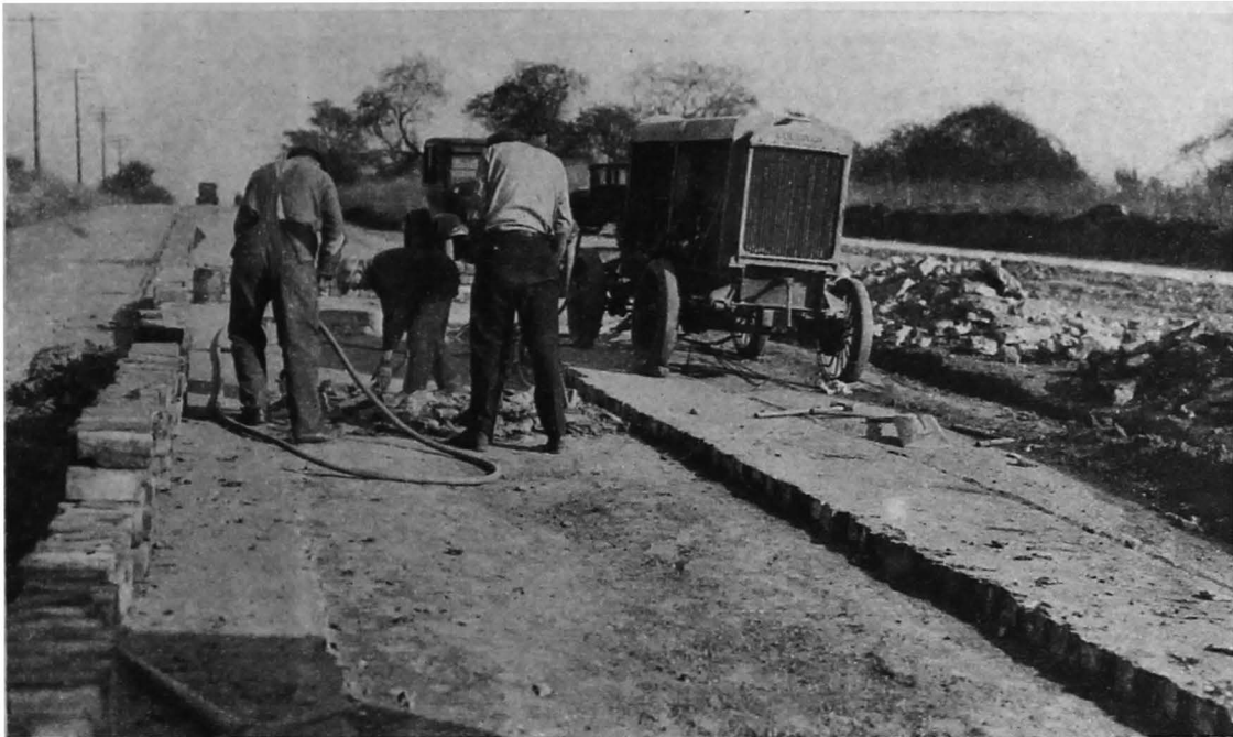
Extensive repairs on Brook Park Road which is planned for reconstruction and widening to 40 feet
