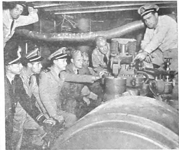
Practical demonstrations on making repairs gives the trainee a good chance to learn
