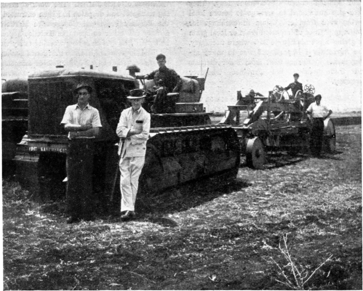
Terracing with a caterpillar D7, 80 H. P. tractor and a road grader.
