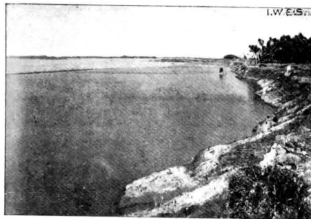
Photo 2606. Deep scour at Dalarghat on Katjuri just downstream of Surua. Looking upstream.
