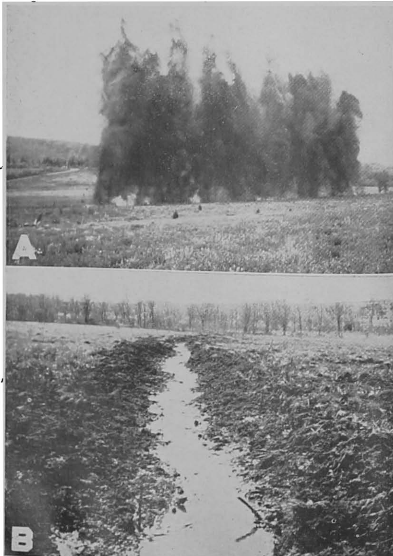
Figure 9. A. Blasting a Ditch Through Swampy Pasture Land. B. Ditch Blasted in Heavy Wet Land.
