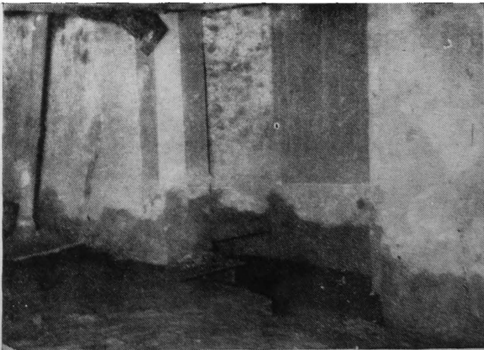
Photographs showing cavitation damage in control tower and conduit
