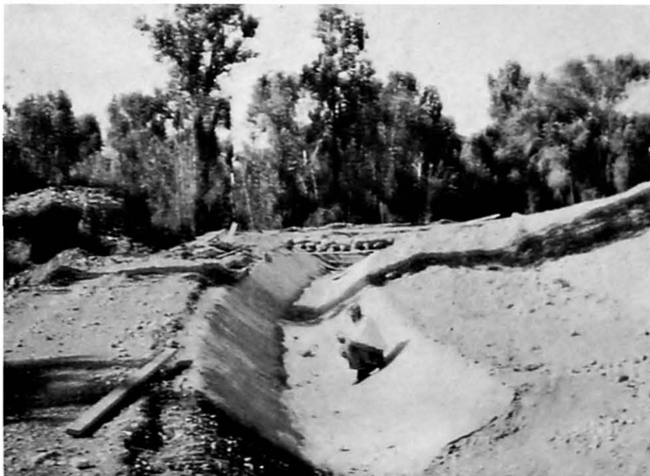
Fig. 2. Richmond Canal Lining Project. Section typifies lining with Gunitite Construction. Supervised by the Soil Conservation Research Division 1948.
