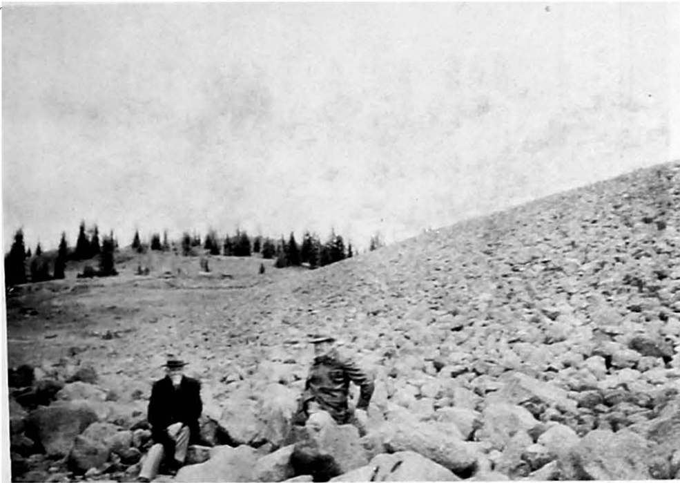
Fig. 3. Spectacle Lake Reservoir, Boulder, Garfield County, Utah Showing riprap of upstream face of dam - 1948.
