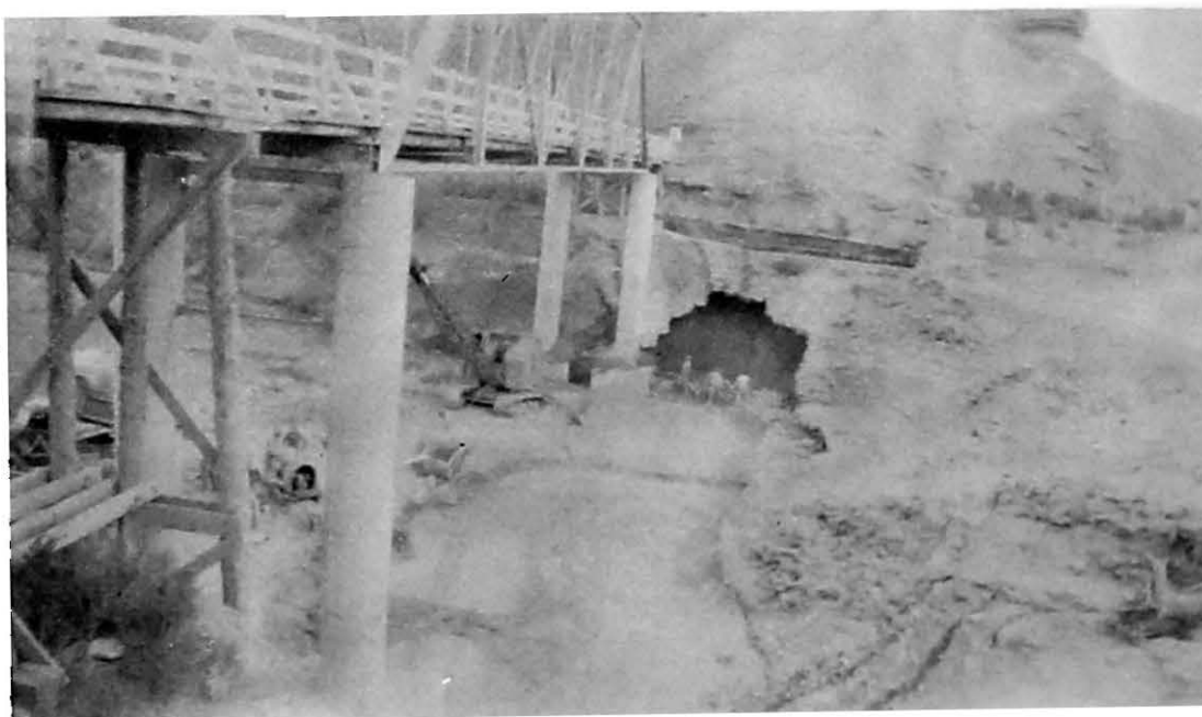
Fig. 6. Hanksville Dam Repair Project. Immediate repair of dam was imperative to prevent total failure of the structure. Looking south, dam has been repaired, with the exception of eroded area on south abutment. Construction supervised by the Utah Water and Power Board.
