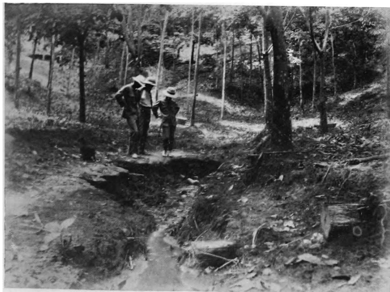
FIG. 37.—SUBSOIL DRAINAGE, A Wash-out.
