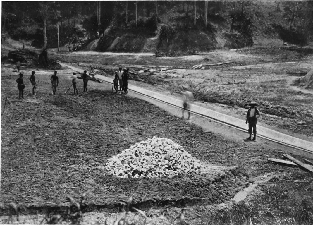
FIG. 106.—LOWER END OF CLUB VALLEY ROAD, KUALA LUMPUR. Showing the central concrete open channel, and a shallow contour drain in the foreground. In the upper portion of this ravine, the concrete channel had to be replaced by a subsoil clay pipe, as shown in Fig. 35.
