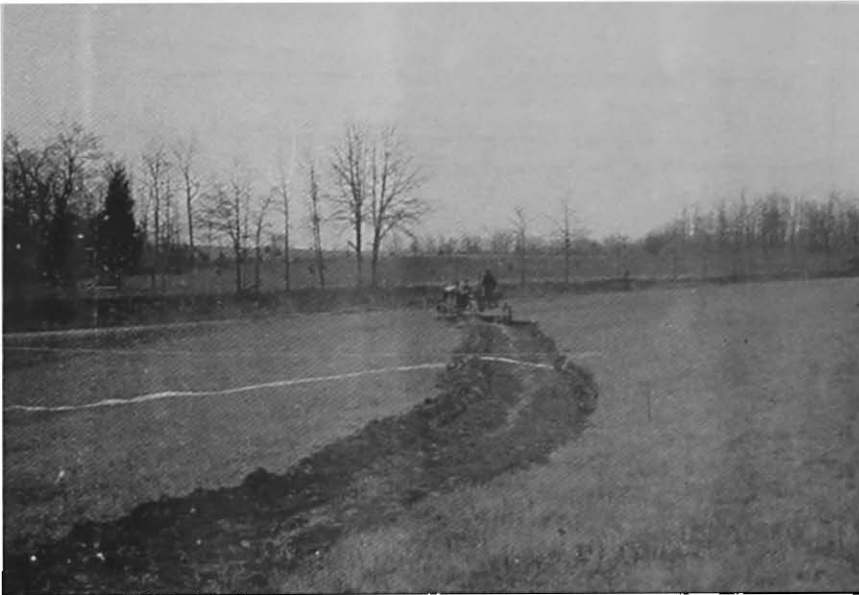
The first cut is made three feet below line of stakes. Care in making this cut is essential if a good terrace is to be constructed with a minimum number of rounds.
