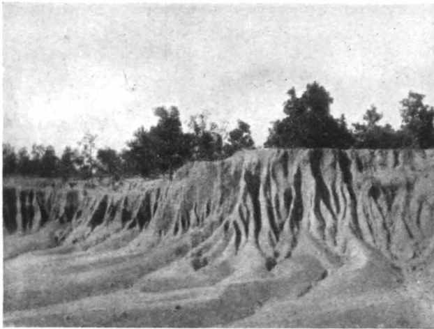
Fig. 19. Scour caused by rain
