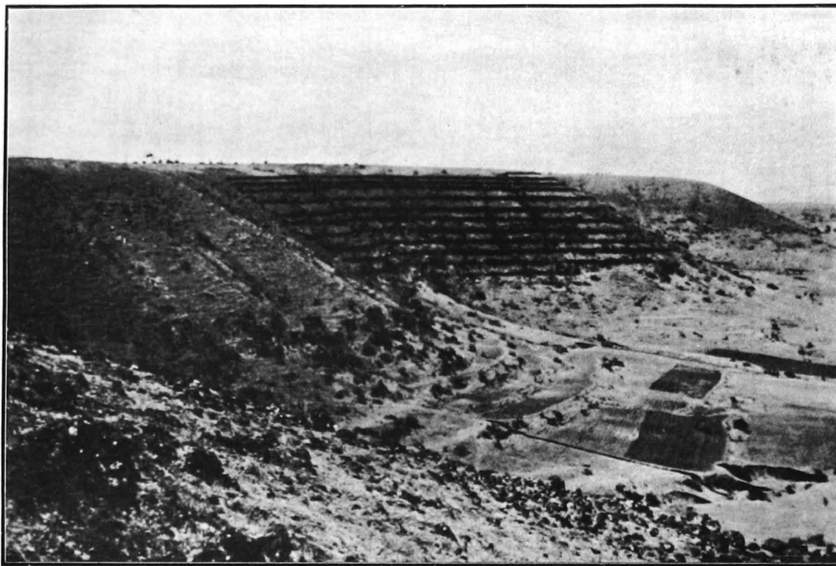
Contour trenching at Nagaon Bari near Dhulia, West Khandesh. Work completed on the further side of the valley. It is proposed to make the flatter bottom of the valley fit for agriculture by means of bunds. The distant trees are along the Bombay-Agra road.
