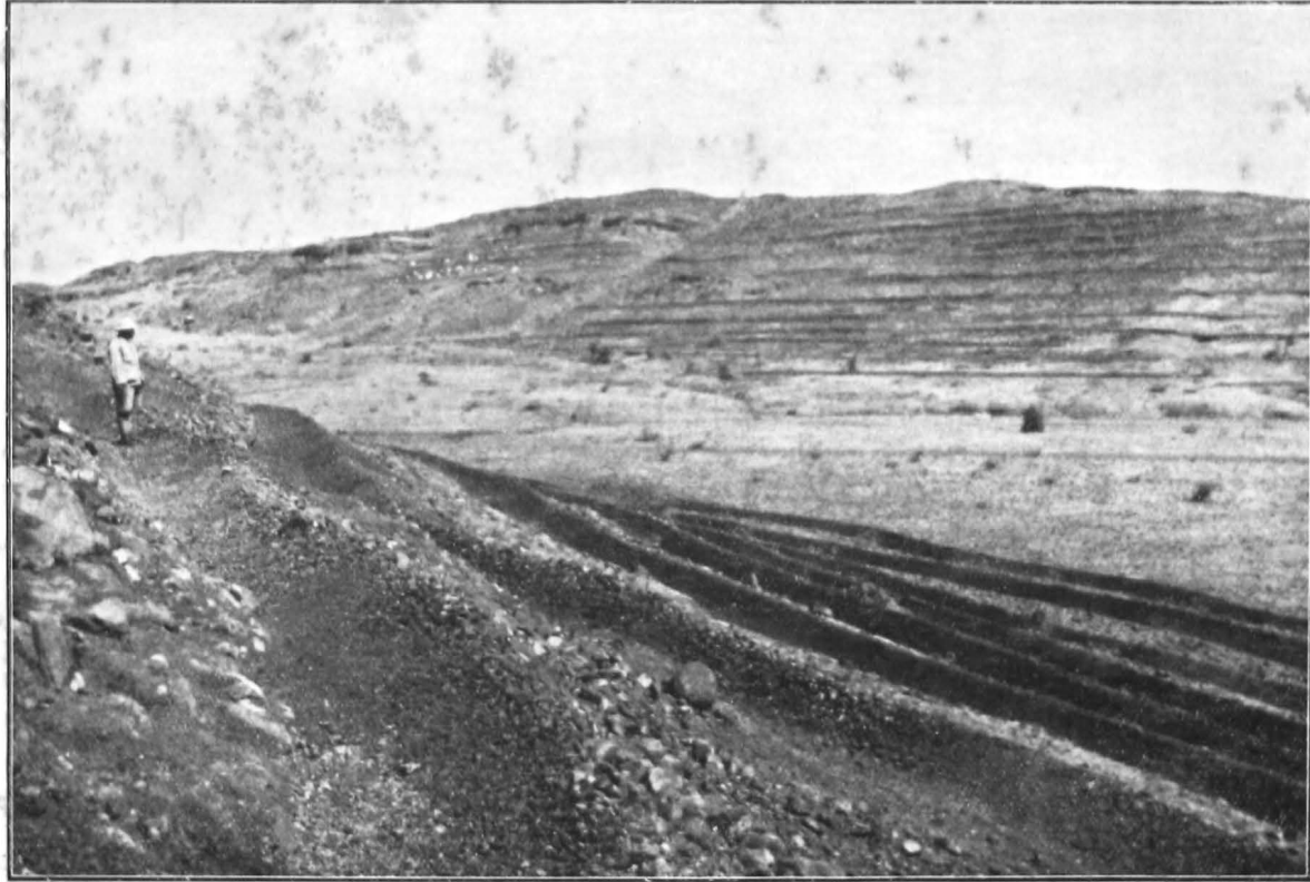
Contour trenching at Nagon Bari near Dhulia, West Khandesh. The average horizontal spacing is 17' but is as close as 9' or 10' near the top of both hill sides shown. The cost is about Rs. 1.8-0 per 100 running feet.
