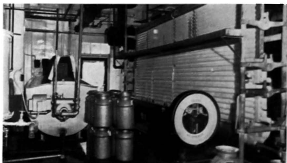
FIGURE 3.—SECTION OF THE PLANT OF THE DES MOINES COOPERATIVE DAIRY MARKETING ASSOCIATION.
