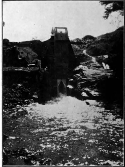
Siphon Spillway at Khadakvasla showing Siphon failing to prime as a result of triangular cut water giving ingress of air, through vertical water diaphragm. Q = 150 Cs. (I. D. R. N. 5.*)
