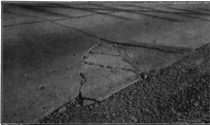
RAPID PROGRESSIVE FAILURE AFTER CORNER BREAK
