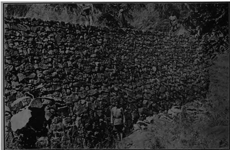
FIG. 17.—Retaining wall on the Subir-Nawapur Road (Surat Dangs). Constructed with Bhil labour. Length 103 ft., height 17\frac{1}{2} ft., and top width of wall 2\frac{1}{2} ft. Cost Rs. 1,121.
