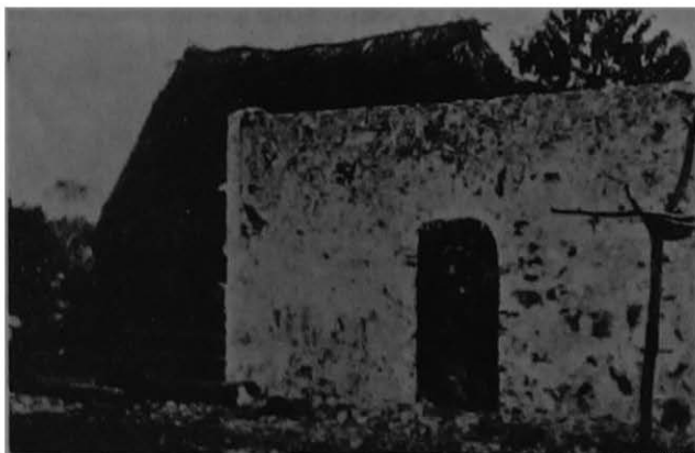
c, Building a masonry house to take the place of the old house.
