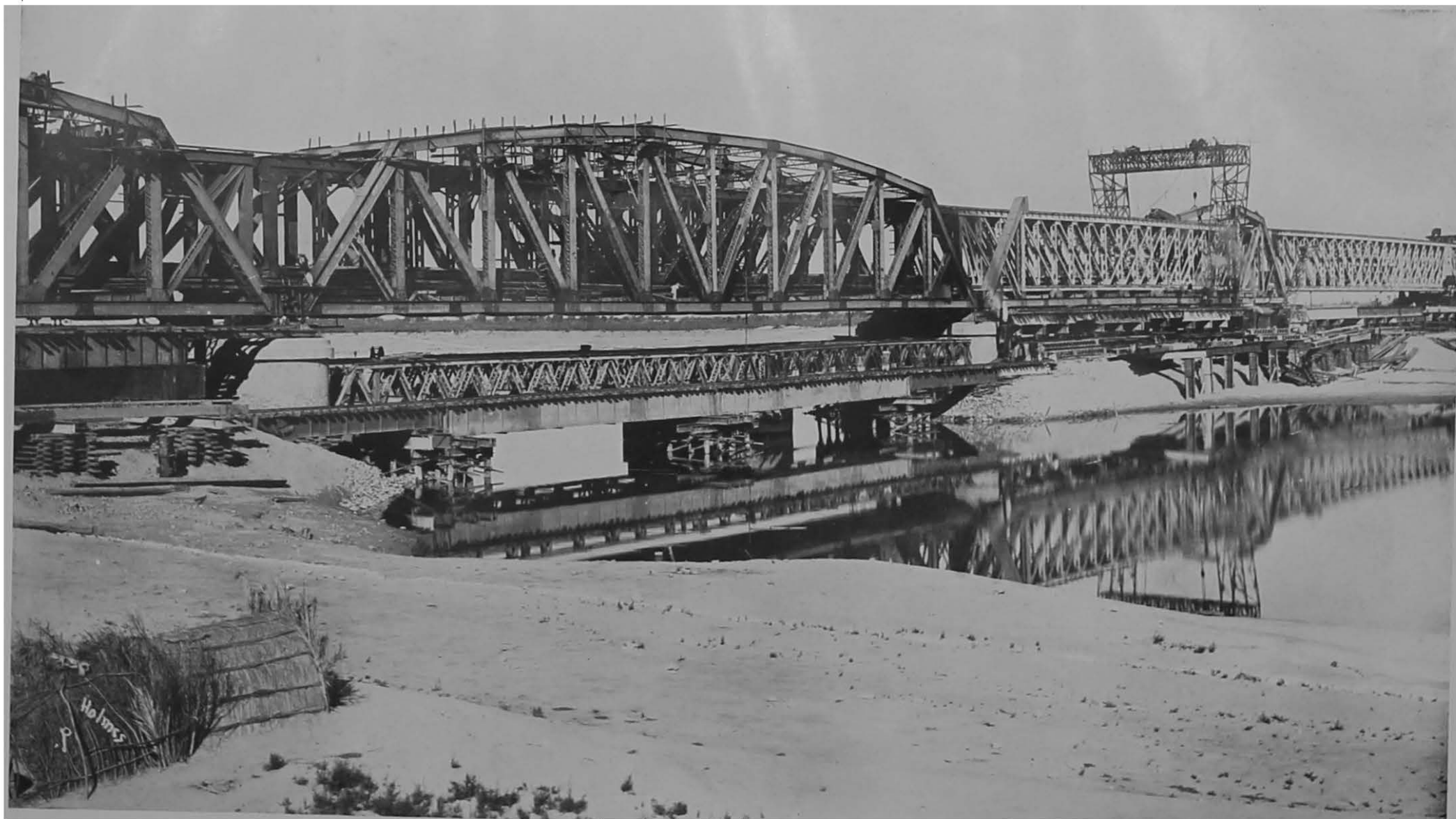
Empress Bridge at Adamwahan. Renewing 8 single track spans with double track spans.
