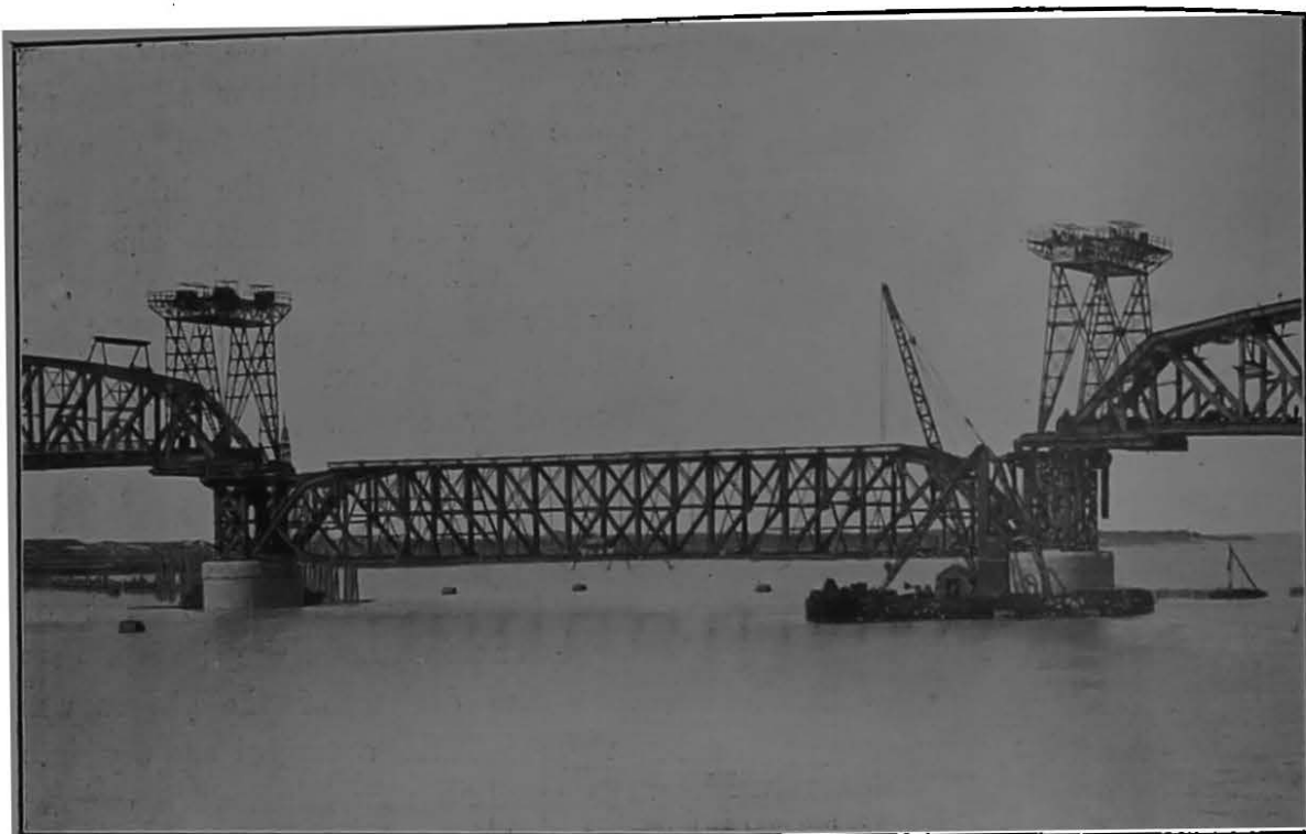
Service Girder in place for erection of last span of Hardinge Bridge.
