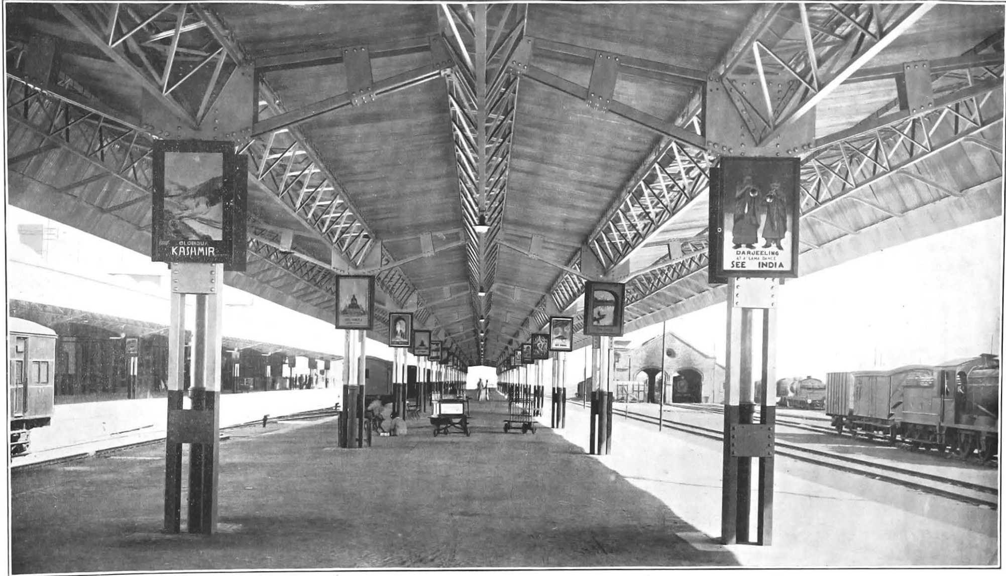
New Platform Roof at Kalka Station built according to Central Standards Office design.
