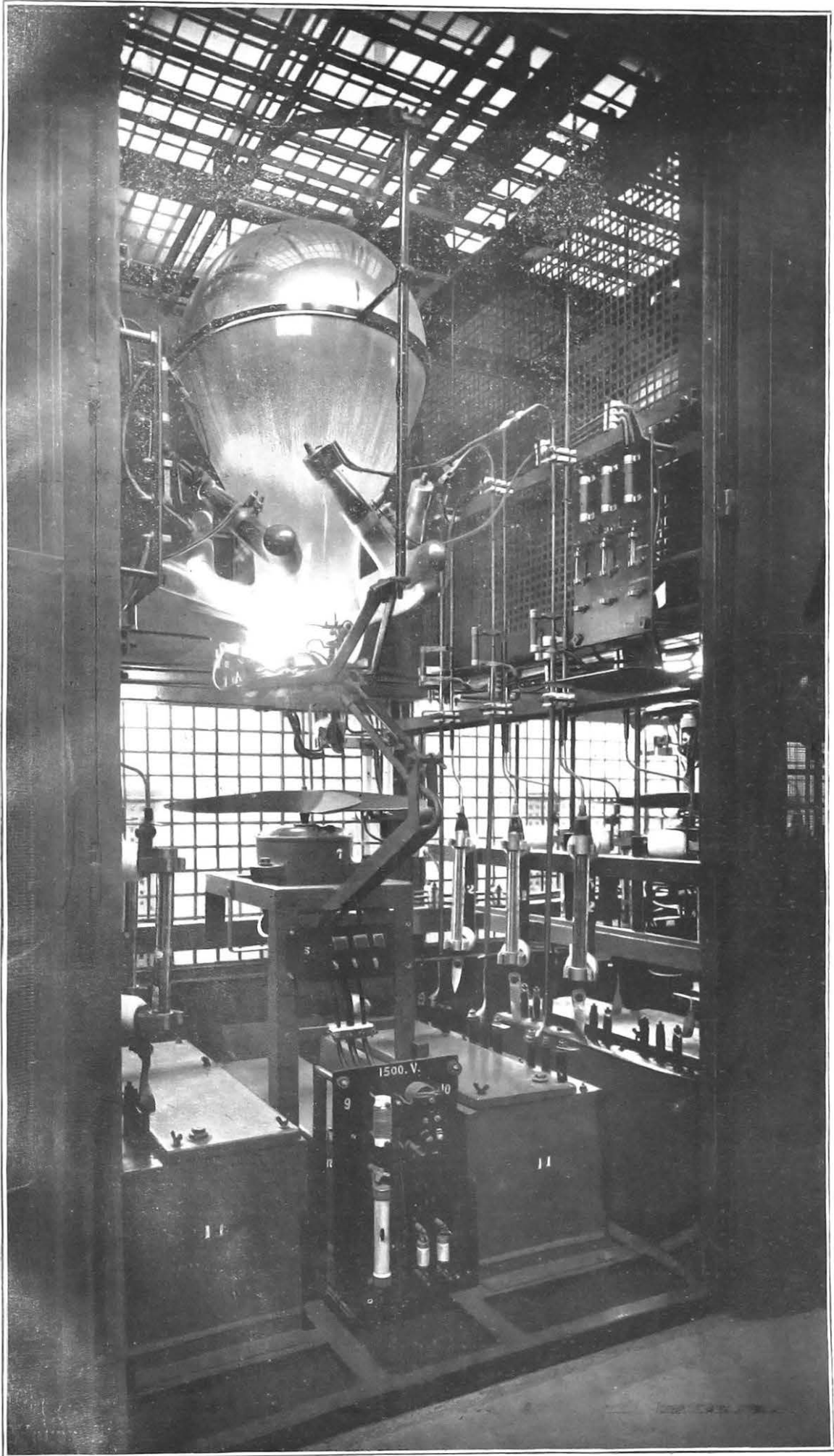
Interior of Electric Sub-station at Bassein Road showing Mercury Arc Rectifiers.
