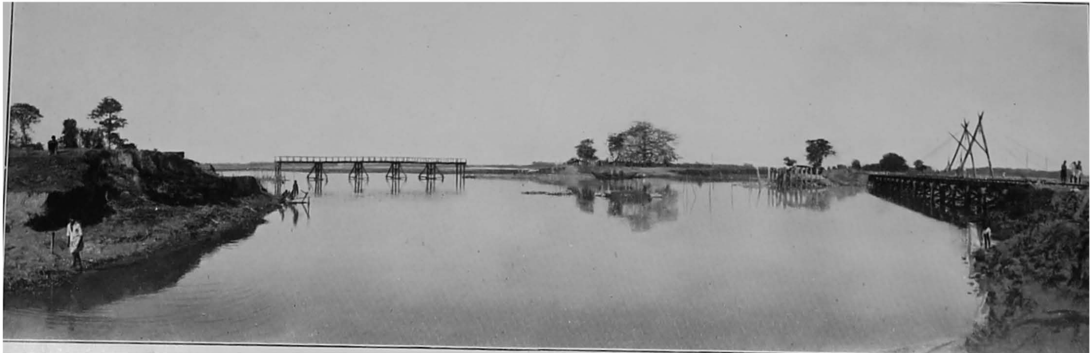
Washout of Ranthali Bridge on Chaparmukh Silghat Railway.
