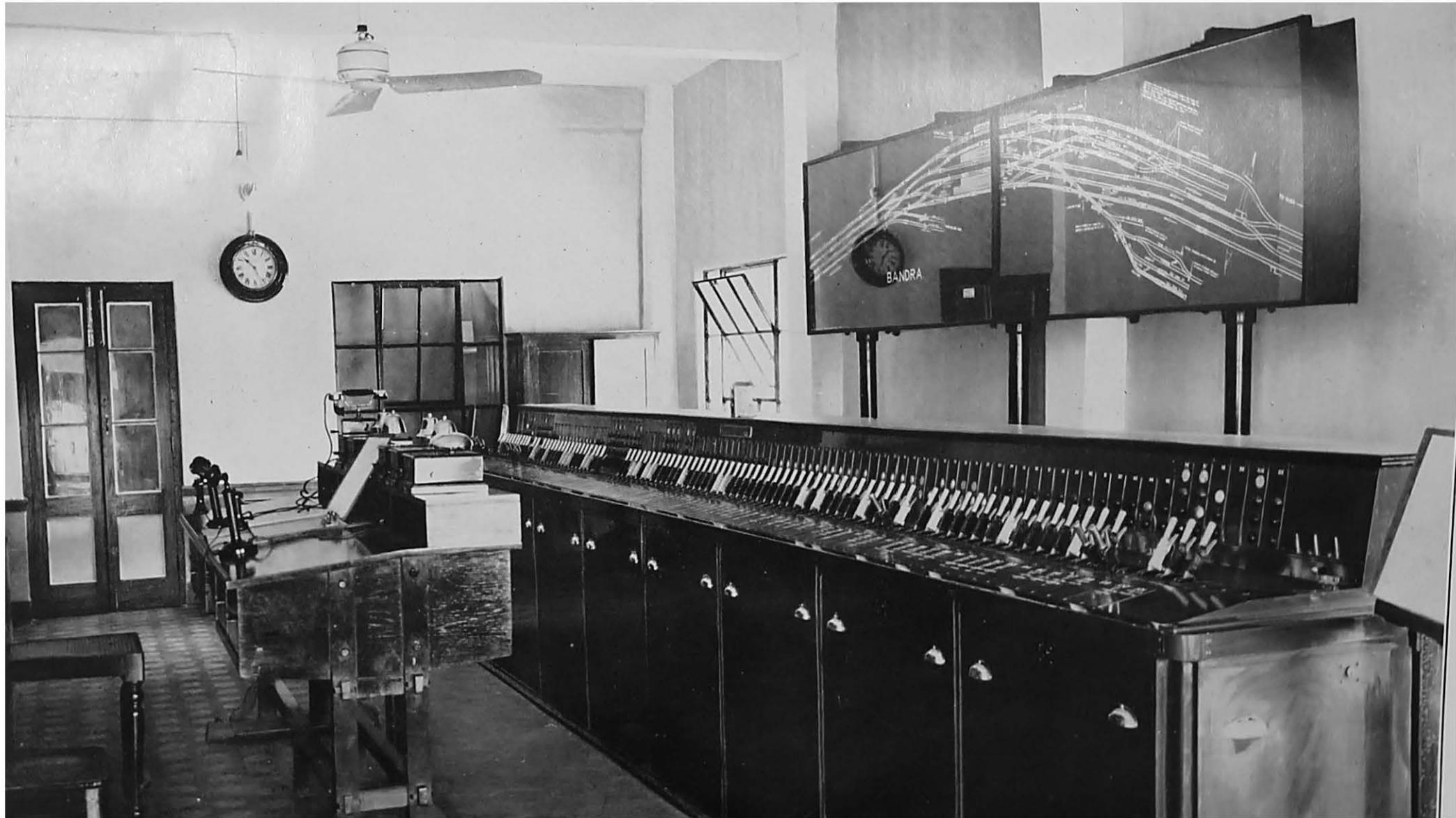
All-electric power signal interlocking lever frame with illuminated signal and track diagram and Block Signalman's table at Bandra Station.
