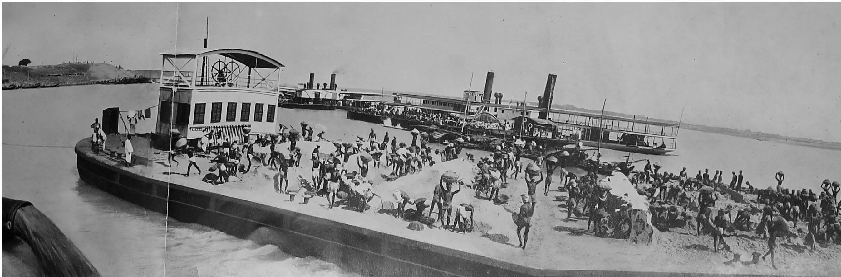
Restoration of the breach of September 1933 of the right guide bund of Hardinge Bridge.
