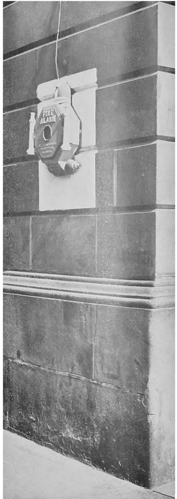
PLATE 33. WALL TYPE FIRE ALARM—GLASGOW.
