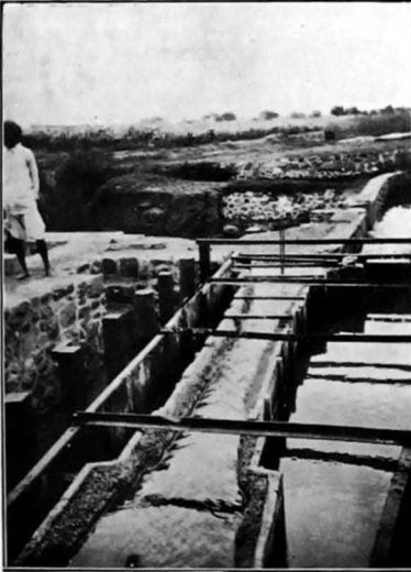
Discharge of 0.83 Cusecs equivalent to 620 Cusecs; new F.S.Q. looking downstream. The view also shows the pointer plate arrangement to observe water levels
