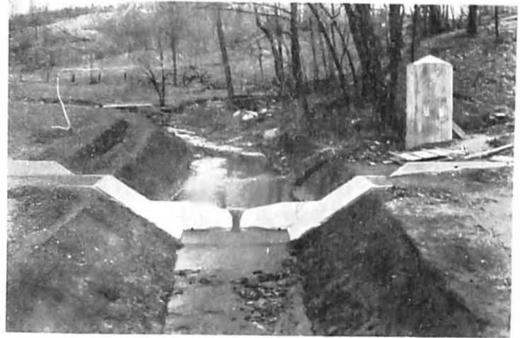
U. S. SOIL CONSERVATION SERVICE FIGURE 25.—Gaging stations on small streams must have a control weir so designed as to magnify stage-discharge relationships for low flows. The control weir shown, known as the Columbus notch, is designed to permit the accurate measurement of small flows. The banks are shaped and sodded to provide stable stage-discharge relationships for high stages.
