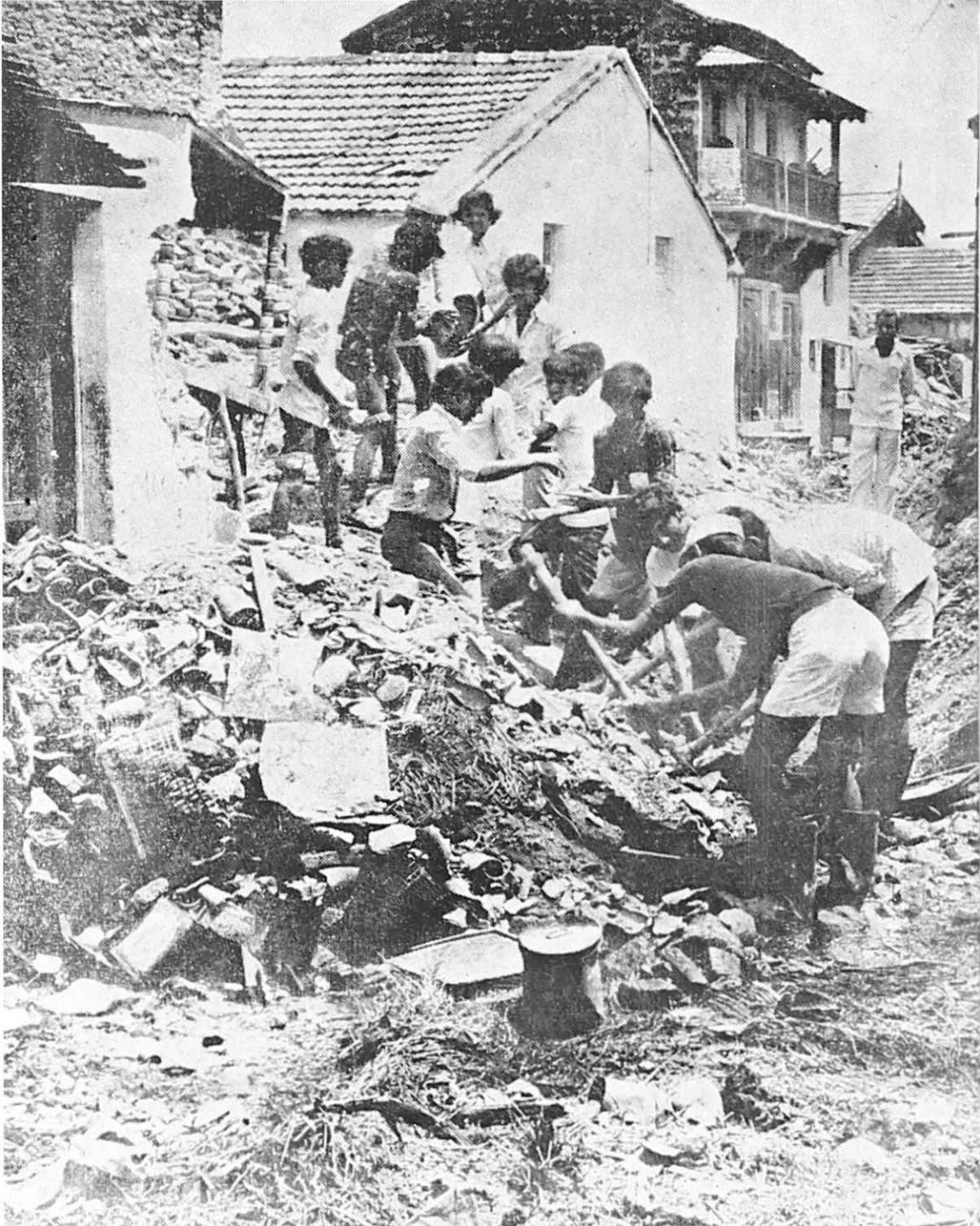
NSS volunteers of the Saurashtra University working in a relief project at Morvi.
