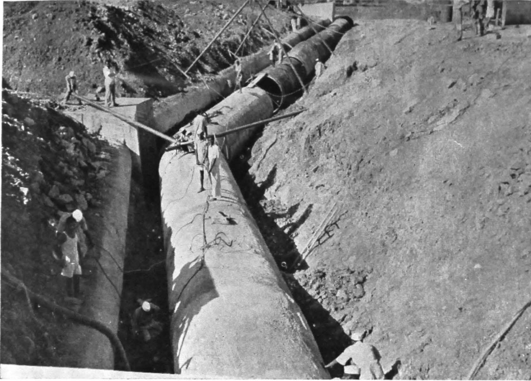
Laying 96" dia. Pipe with a Sharp Bend Under Ground in Santa Cruz Aerodrome
