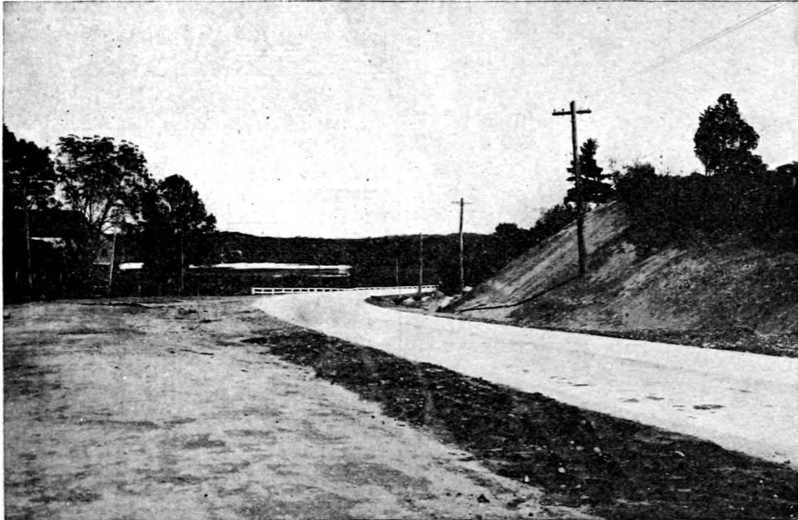
A CONCRETE SECTION OF THE BOSTON POST ROAD WHICH REPLACES AN OLD WATERBOUND MACADAM SECTION. IN THE NEW CONSTRUCTION, THE BANK AT THE RIGHT HAS BEEN CUT BACK TO EXTEND THE SIGHT LINE
