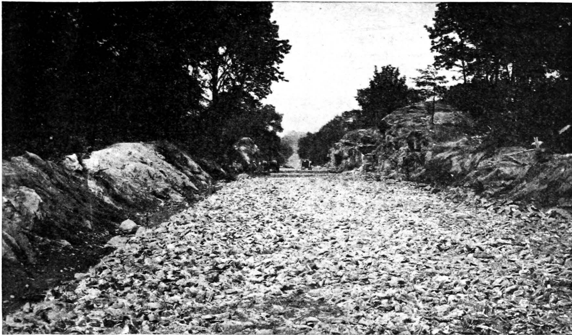
THE BOSTON POST ROAD IS CLASSIFIED AS A TERMINAL HIGHWAY. BECAUSE OF THE IMPORTANCE OF ITS TRAFFIC, IT IS ENTITLED TO THE HIGHEST TYPE OF PAVEMENT OF THE HEAVIEST DESIGN. THIS VIEW SHOWS A STONE FOUNDATION LAID AS A PART OF THE RECONSTRUCTED HIGHWAY NEAR GREENWICH
