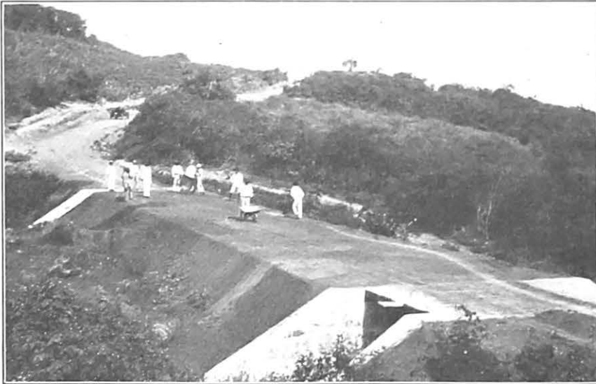
Figure 8.—Grading and filling on the road from Santa Cruz to Torre, Pernambuco
