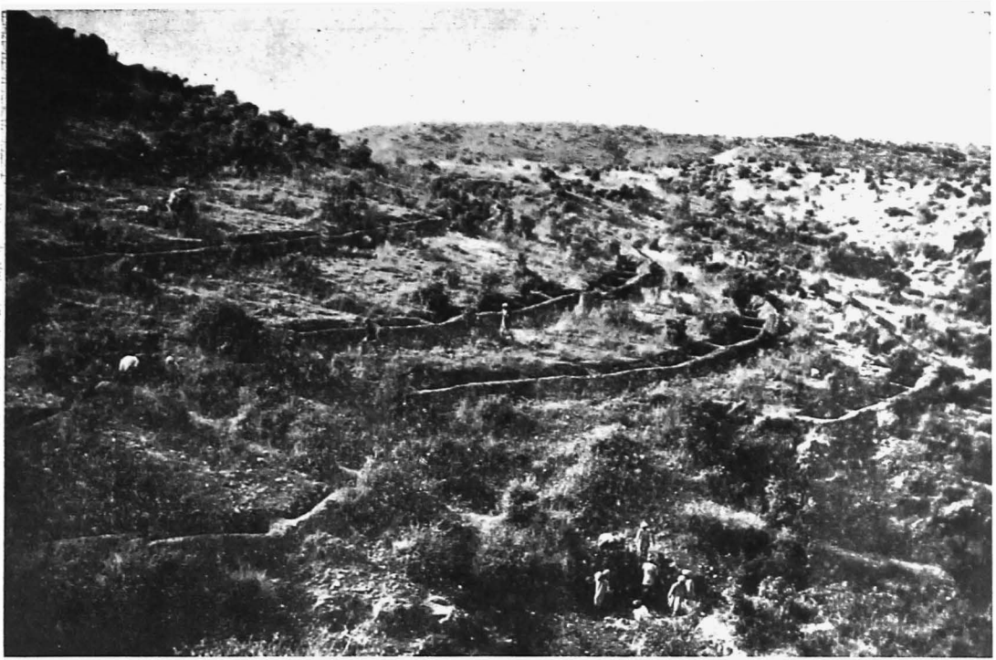
This shows that contour trenches are not straight lines, but must be laid out accurately level so as to catch maximum of water. Squad below is building a checkdam in the nala bottom.
