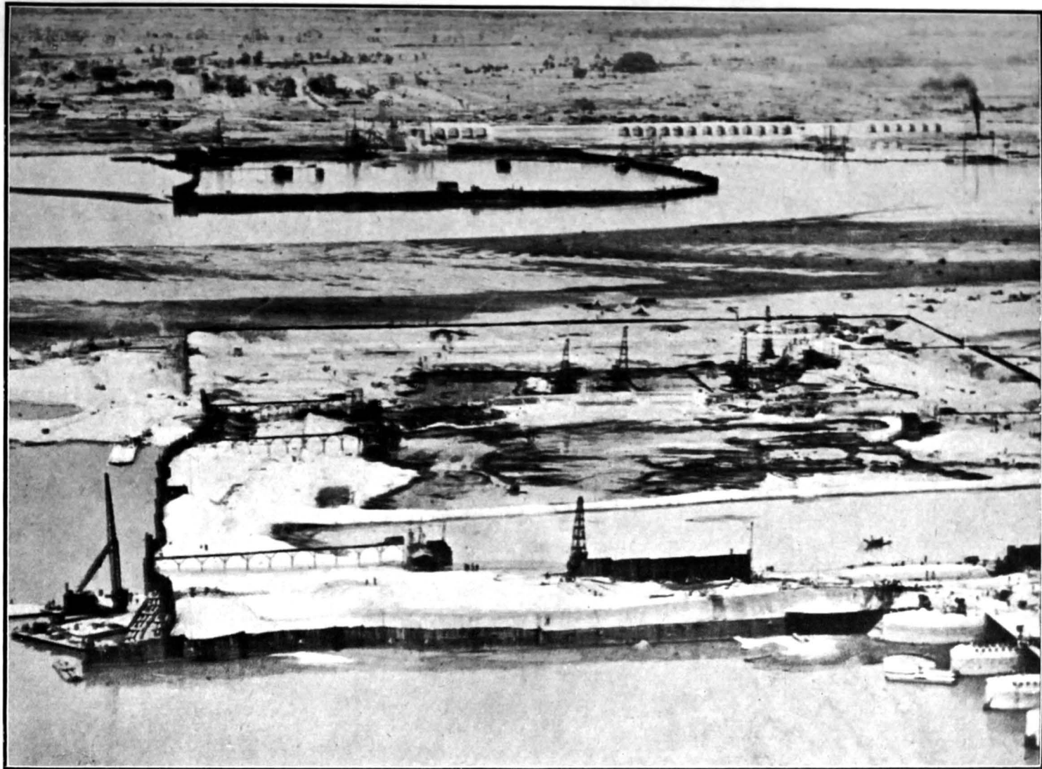
Right Bank (in distance) & Left Bank (in foreground) Cofferdams, Head Regulators of Dadu, Rice & North Western Perennial Canals are seen in distance.
