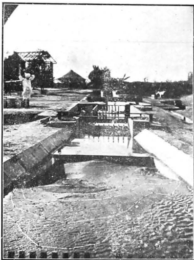
662. Showing heavy scour which would have occurred downstream of the Tando Mastikhan Fall (Rohri Canal, Sind) with 1 in 10 divergences without remodelling.
