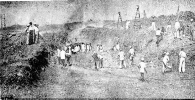
Gangapur Storage scheme:—Picture shows excavation of a rock to cut off trenches designed to let out the surplus water.
