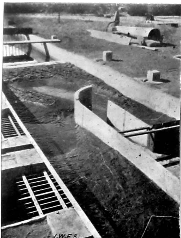
Photo 489. Escape at the nose of the Divide Wall—facing away from the canals—looking upstream.
