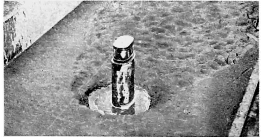
Scour round Bridge Pier
