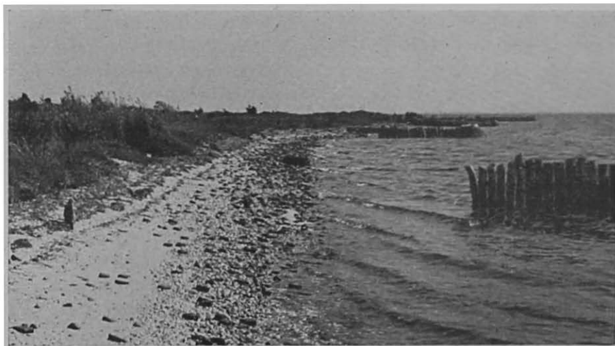
Figure 39. On the south shore of Long Island. The waves have cut away the shoreline in spite of the protective works and the piling.
