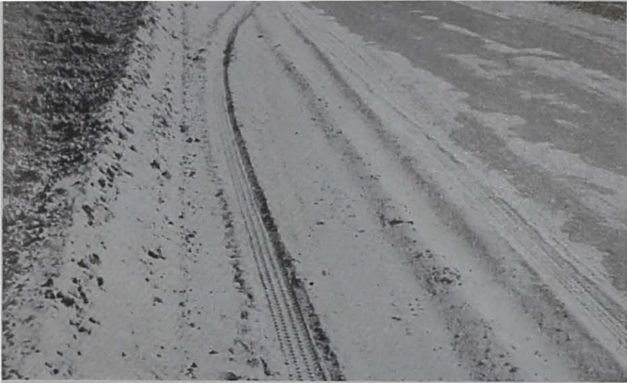
Figure 20. Potato rows slope toward highway. After heavy rains the road must be cleared of sand with a scraper, as shown here. The finest soil particles have been lost entirely. Clearing is costly to the public, including farmer taxpayers.
