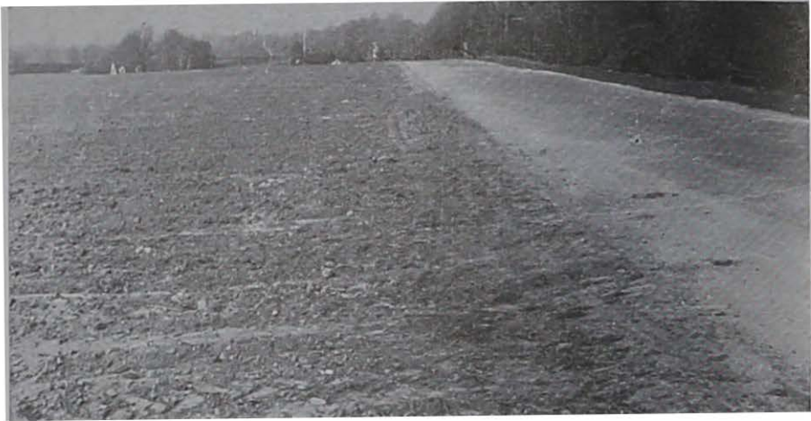
Figure 19. Right-of-way up to actual hard surface of highway being cropped. Destructive blowing and washing may result from this practice.
