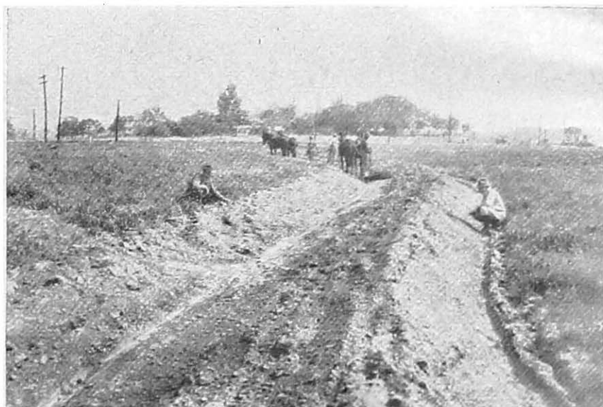
FIGURE 24.—Terrace construction with a plow and V-drag. It requires considerable work to construct satisfactory terraces with this type of equipment.
