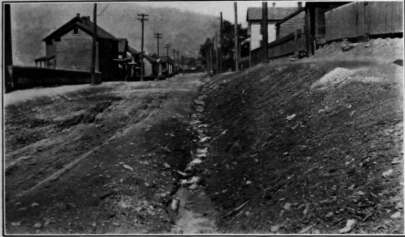
AN OPEN DITCH ALONG NEW STREET, PROSPECT.
