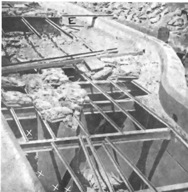
View of fan drift roof which was destroyed by first explosion. The four deceased fell into fan drift at points XX. Note the temporary seal over fan evasee at E.
