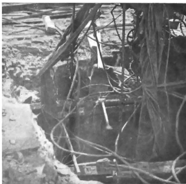
View showing kee beams and mouth of upcast shaft after wrecked cage had been removed.
