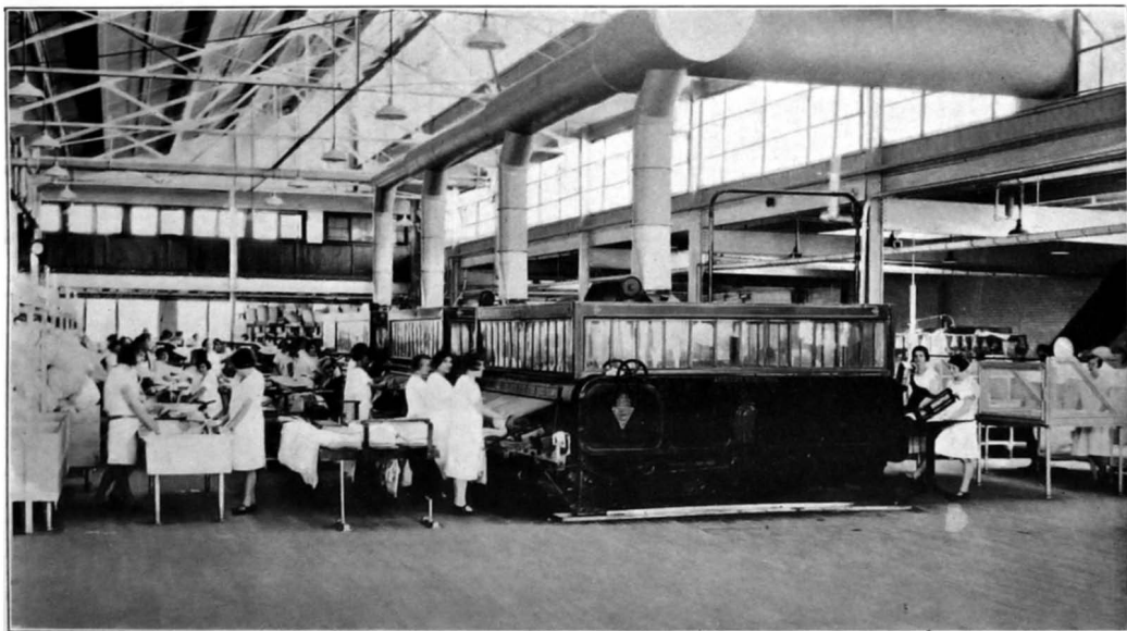
PLATE 2.—THE HEAT FROM THE FLAT-WORK IRONERS IS CARRIED OFF
