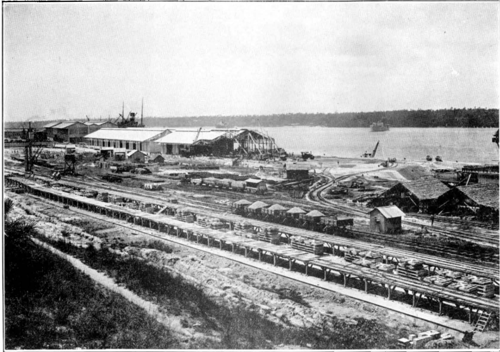
KILINDINI HARBOUR WORKS. GENERAL VIEW OF SHEDS ON BERTHS Nos. 3 AND 4 UNDER CONSTRUCTION.
