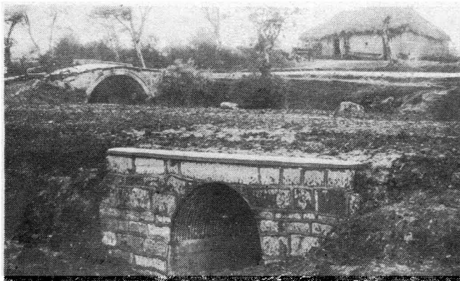
上：安徽段內半圓綑鐵管涵之洞 Above—A Semi-circular Corrugated Steel Culvert—Anhwei Section
