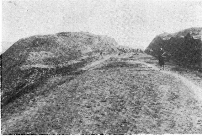
程工山開近附城宜內段徽安：上 Above—Rock Excavation near Sūancheng —Anhwei Section
