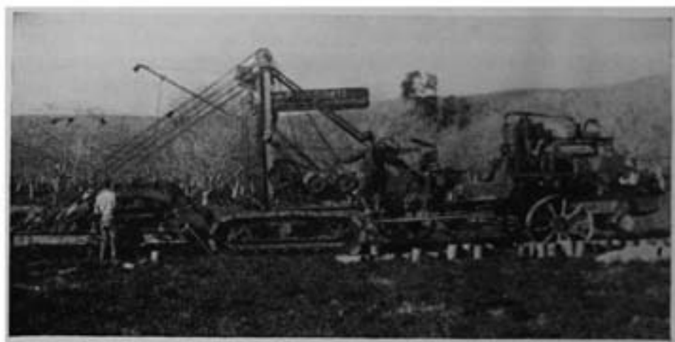
Drainage contractors use excavators which dig trenches rapidly and accurately at usually less cost than the work can be done by hand.
