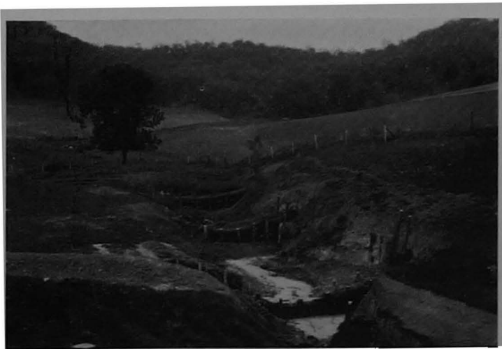
FIGURE 20.—Inexpensive wire and post check dams to curb severe gullying on the Coon Creek Watershed near La Crosse, Wis.
