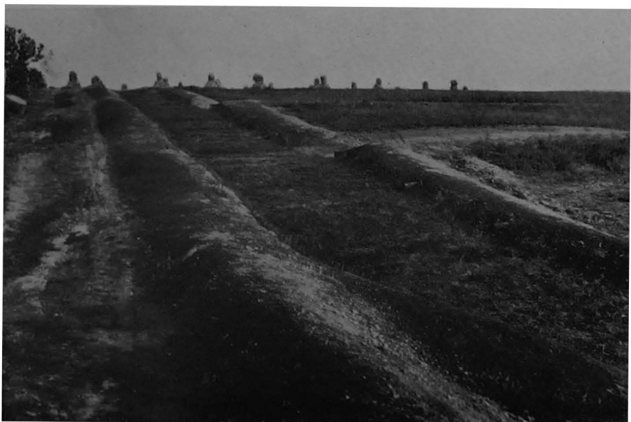
Sodded terrace outlets, employed by the LaCrosse, Wis., project, to conduct water safely from terraces to lower levels.
