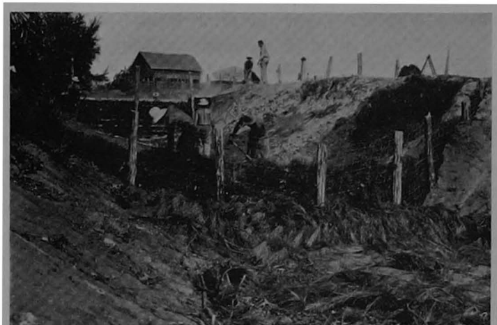
FIGURE 22.—Members of the Civilian Conservation Corps building an inexpensive wire and post dam to curb gully erosion, near Minden, La.
