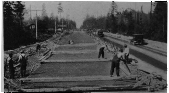
CONCRETE ROAD CONSTRUCTION IN WASHINGTON. ONE 20-FOOT LANE IN USE WHILE A SECOND LANE IS UNDER CONSTRUCTION
