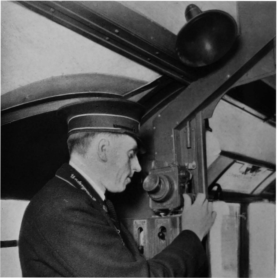
Fig. 70. A guard in telephonic communication with his driver, the loud-speaker in this case being fixed in the roof.
