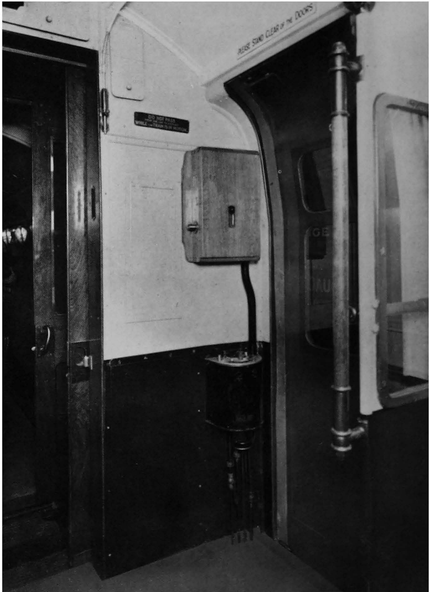
Fig. 68. This equipment includes a signal light which appears only when all doors are closed. Until then the guard cannot operate the bell signal to the driver to start.
