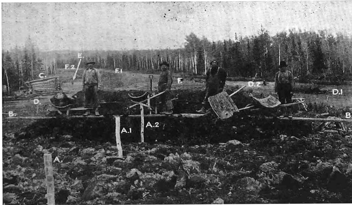
A, A1, A2—STAKES OF ENGINEERS TO SHOW GRADE LEVEL ; B, B1—HEWED TREE-PLANKS FOR RUNWAY ; C—STATION-MEN'S SHACK ; D, D1, D2—SHOWING EXCAVATIONS MADE ; E—AN "ISLAND" TO INDICATE CLASSIFICATION ; F, F1, F2—GRADE BUILT TO LEVEL
